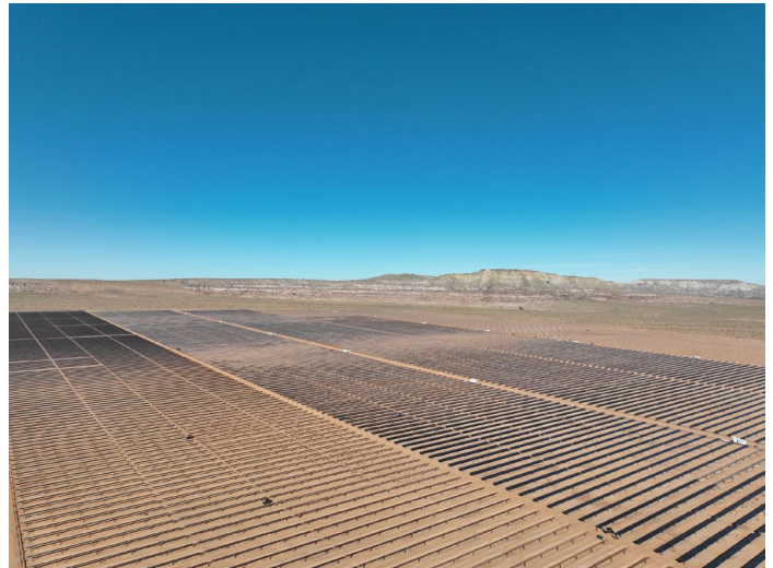
Red Mesa is a 70-MW solar farm developed by NTUA. This photo shows the array under construction. Photo by Glenn Steiger, NTUA
