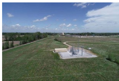
Saginaw Chippewa Indian Tribe of Michigan’s substation supporting Tribal utility operations. Photo by Brian Smith, Saginaw Chippewa Indian Tribe of Michigan
