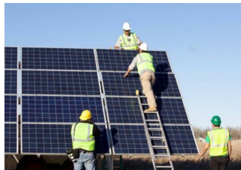
Leech Lake Tribal College students gain hands-on workforce experience installing a solar PV array. Photo by Eugene Strowbridge, Leech Lake Band of Ojibwe
